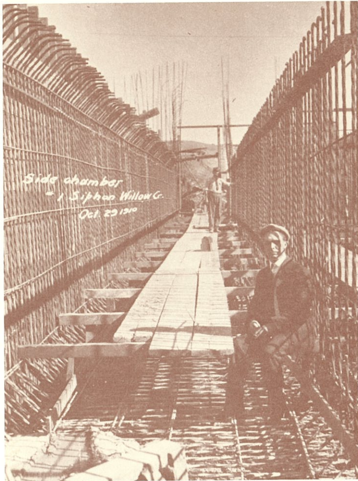
Construction of side chamber of Willow Creek Siphon (Courtesy of Special Collections, Meriam Library, California State University, Chico)
