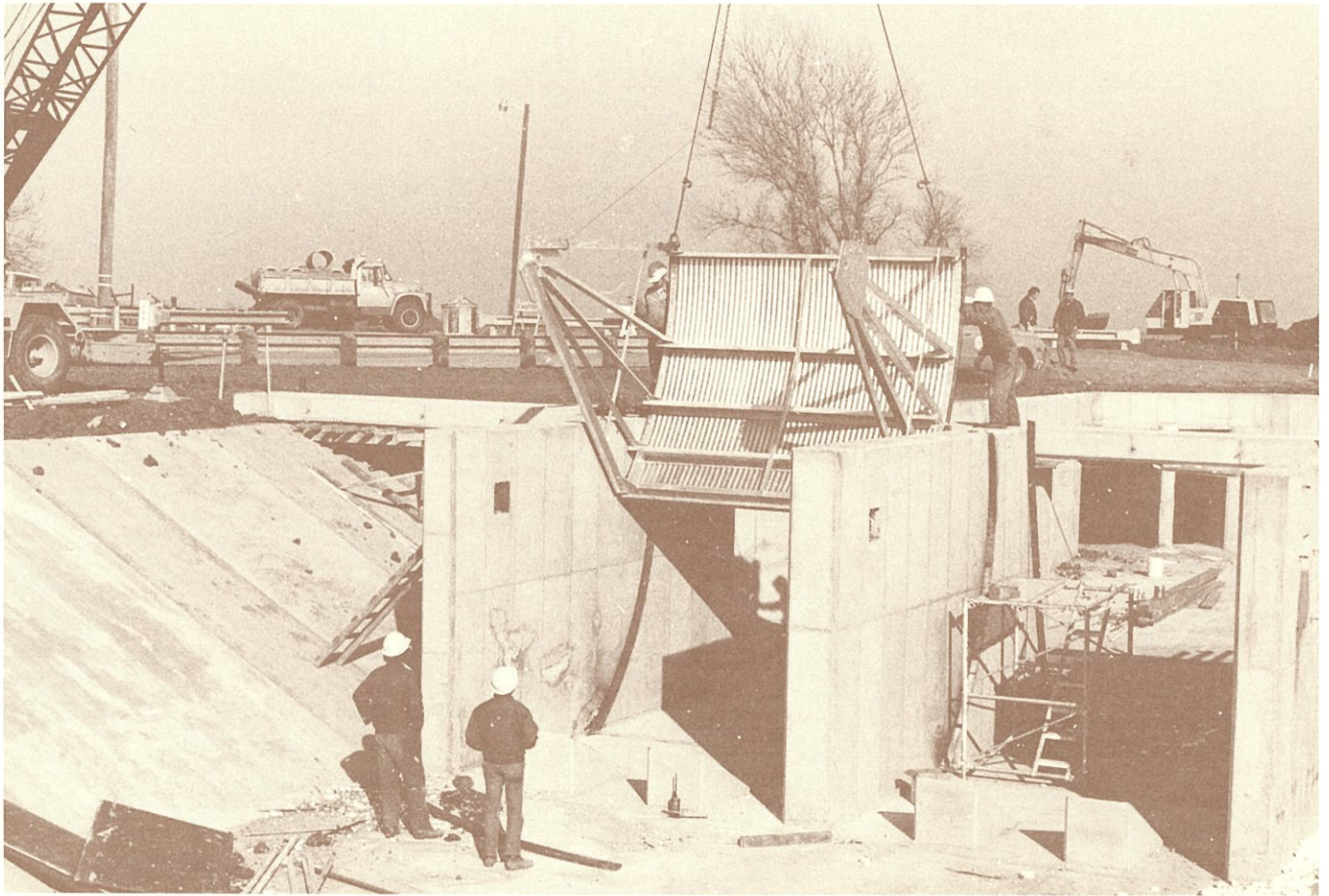
Glenn-Colusa Irrigation District crew installed radial gate (designed and constructed by District forces), at Freshwater Check and Siphon, to complete enlargement and modernization of check and siphon structure
