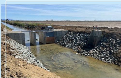
Photos above: Pouring concrete floor and curtainwall on new check structures. Completed new check structure.
